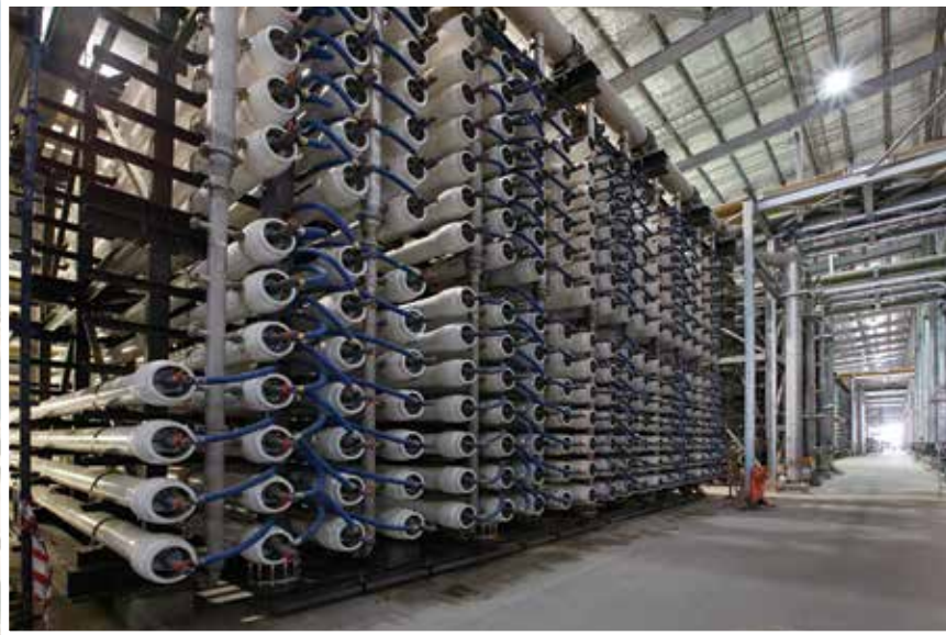
THE REVERSE OSMOSIS MEMBRANES INSIDE THE SYDNEY DESALINATION PLANT.
